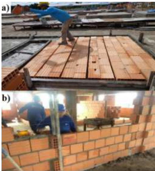
Figure 2: a) Assembly of ceramic blocks for the execution of precast walls; b) Execution of masonry in a conventional manner.
