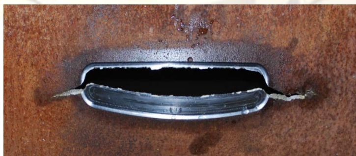
Fig. 3 .Corroded pipe after burst test [ 8]
