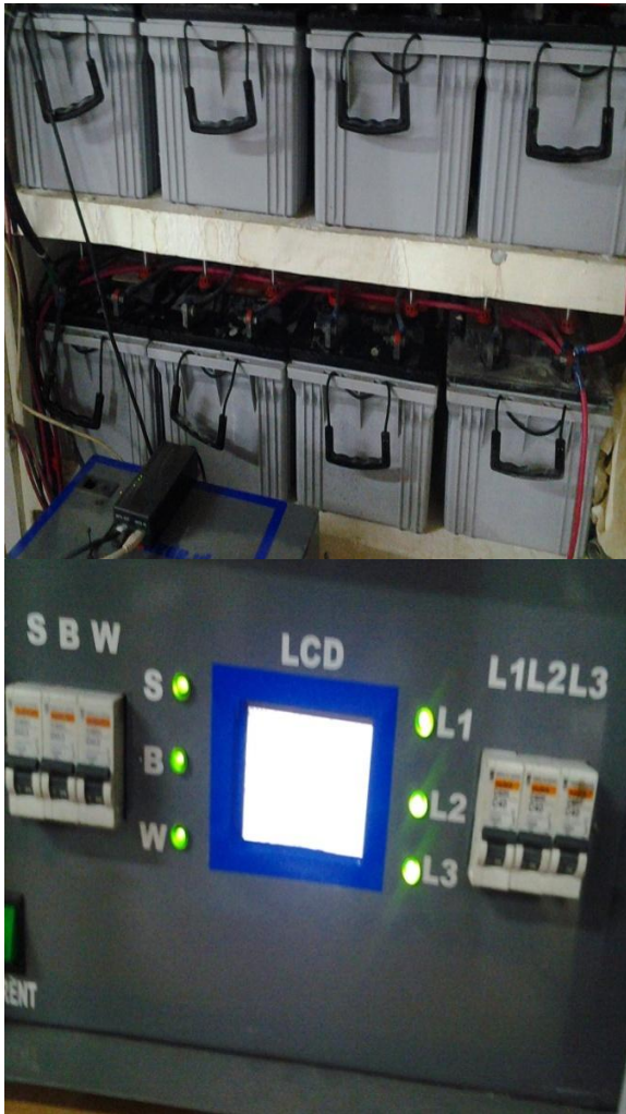
Fig: 9 battery storage unit & controller.
