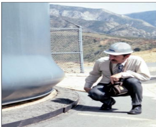
Fig 1 Elephant-foot buckling of a tank wall Sloshing liquid can damage the roof and the top of tank wall as
