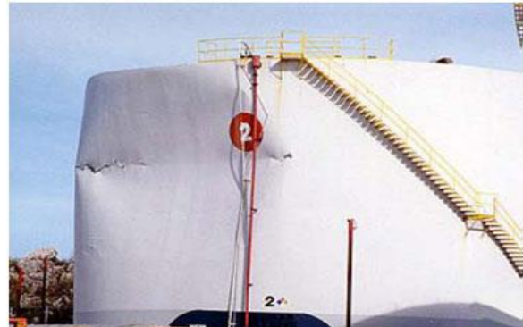
Fig 2 Sloshing damage to upper shell of tank Base shear can overcome friction causing the tank to slide. Base uplifting in unanchored or partially anchored tanks can damage the piping connections that are incapable of accommodating vertical displacements, rupture the plate shell junction due to excessive joint stresses, and cause uneven settlement of the foundation.
