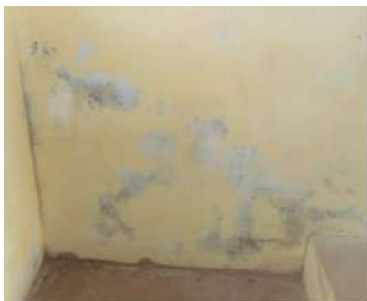
Fig -2: Peeling of distemper in wall
