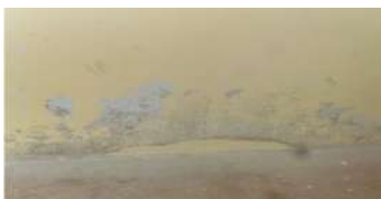
Fig -3: Peeling of distemper and exposure of plaster
