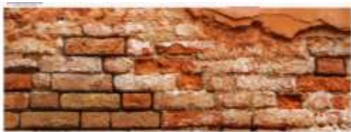
Fig -1: Efflorescence in Brick wall
