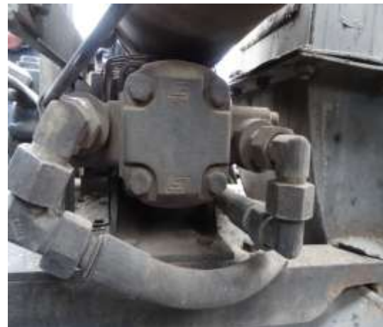
Fig. 11. Hydraulic motor, driving the WS-104 pump
