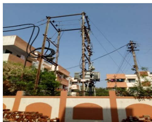
Fig - 1 Transformer in Prem Nagar Colony Substation.
