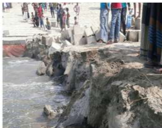
Figure 1.5: Slope failure after permanent wave protection, March, 2017
