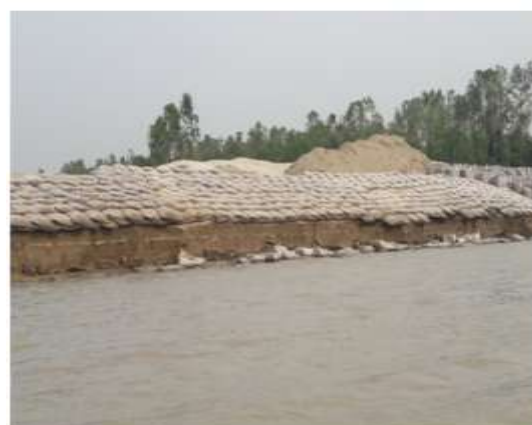
Figure 1.4: Slope failure after temporary wave protection, May, 2016
