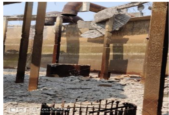
Fig. 9 Column and Slab reinforcement is exposed due to Chlorine attack
