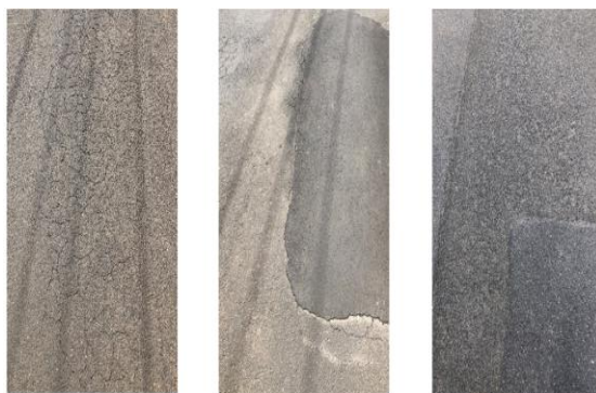
Fig. 2 Sample of pavement distresses on the selected road surface
