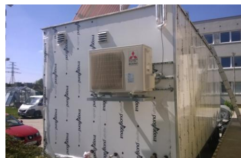
FIG. 8 View of a mobile laboratory - heat source - heat pump [Photo source: authors]
