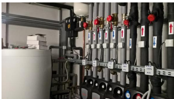
FIG. 4 Connecting a non-functional solar circuit to a bivalent hot water tank [source: authors]
