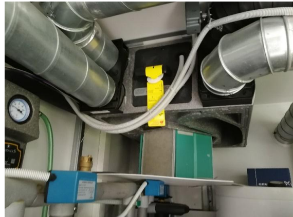
FIG. 12 View of the recuperation ventilation unit [Photo source: authors]
