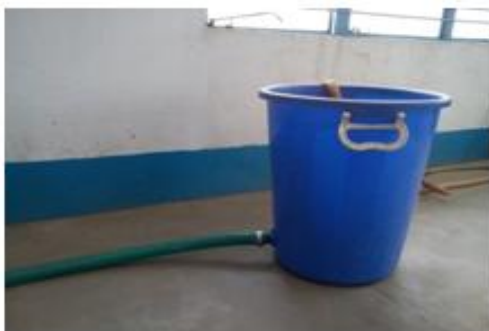
Picture -1 Header Tank
