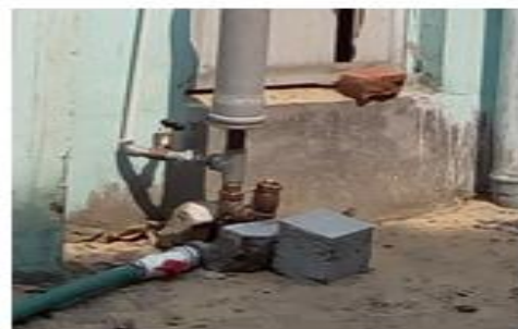
Picture-3 Pump Basement
