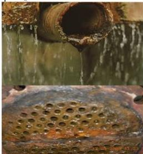
Figure 1: Fouling in Cooling Tower
