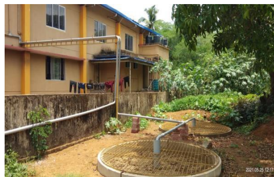
Fig. 7 Roof-Water Harvesting for Town Hall Kumta
