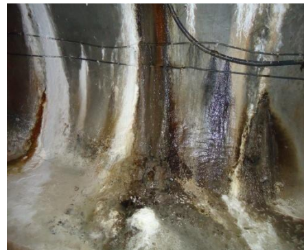
Figure 2 White Leachate Deposit in the Concrete gallery
