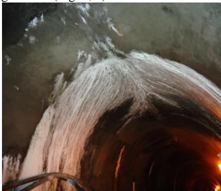
Figure 1 White Leachate Deposit in the Concrete gallery
