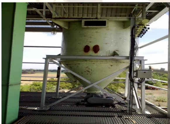
Fig.6. Before implementing cyclone separator in between bag filter and blower
