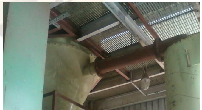
Fig.7B. After implementing cyclone separator in between bag filter and blower (With cyclone separator, duct and bag filter)
