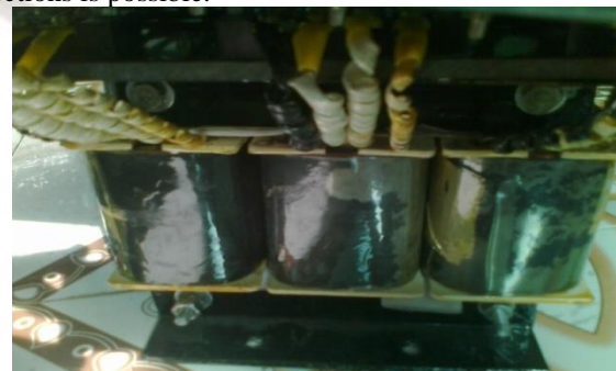
Fig.1 - The three phase transformer with tapping.
