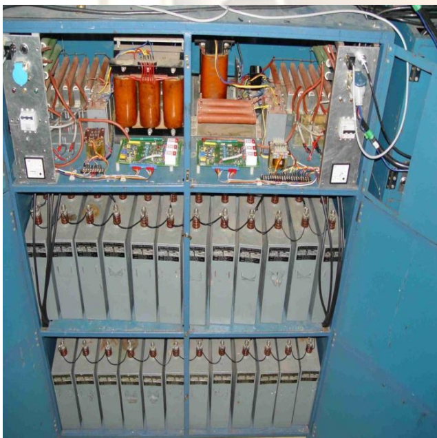
Fig. 3. Power supply capacitor bank
