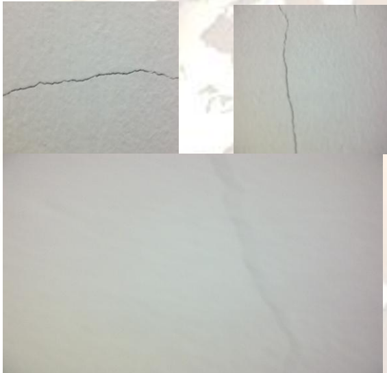
Figure 1: Presence of crack on a wall. (This shows the presence of crack in a wall as its appearance varies from one wall to another)
